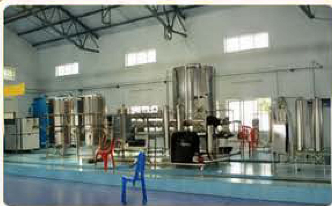
SS Mineral Water Plant
